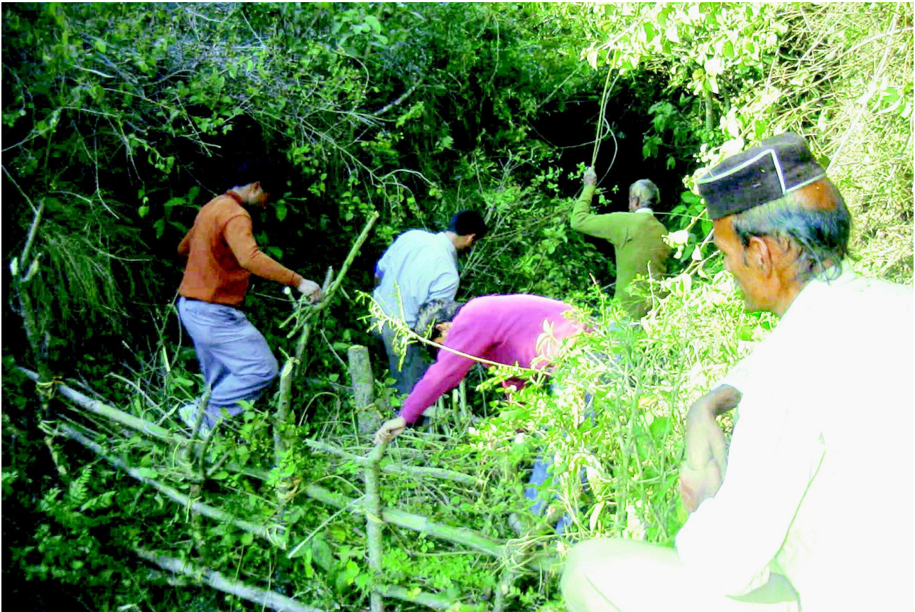
Figure 6 : Construction of a brushwood checkdam in progress (Source : Down to Earth, November, 2008)
