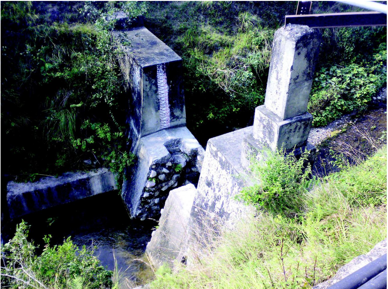
Figure 1: The nullah that runs through Kartar Chand Rana village, Kuhan (Source : Down To Earth, November 2008)
