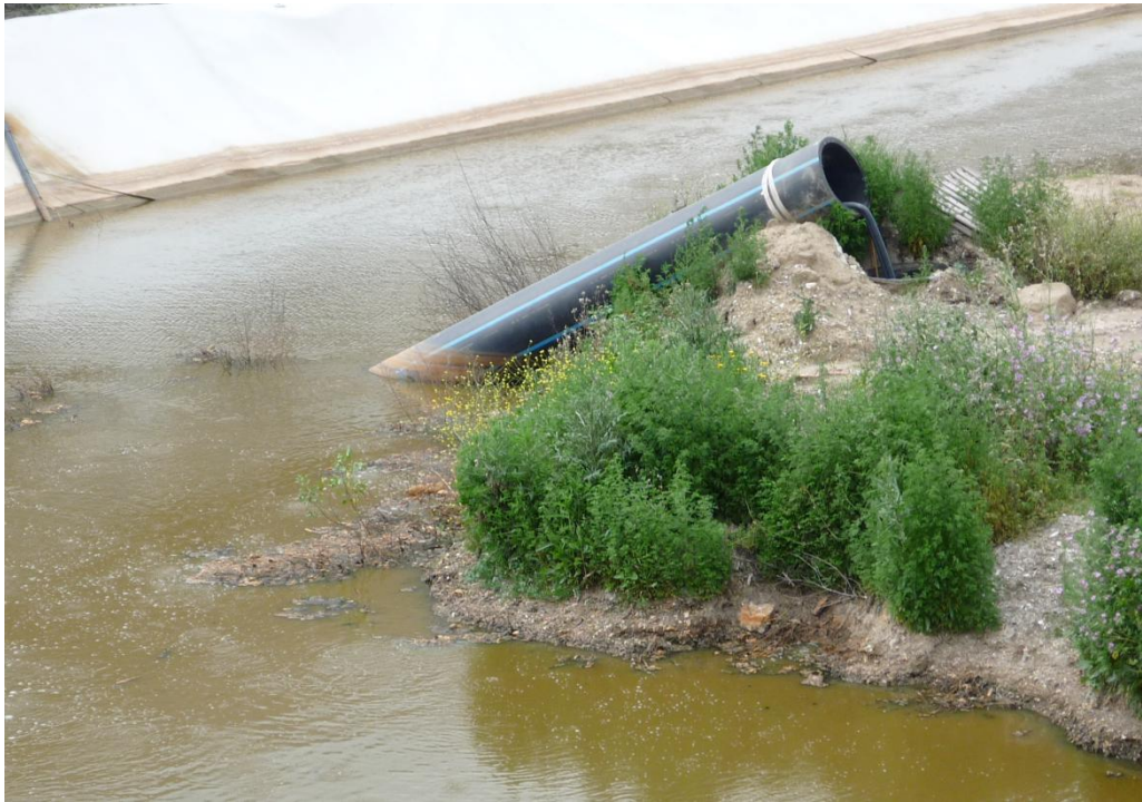
Figure 13: Buried landfill from the Uttaro dumpsite, showing obvious non-conformity (leachate and a broken chimney for gas expulsion) to safety requirements
